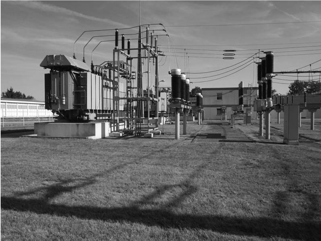
FIGURE 1.15 Substation power transformers.
